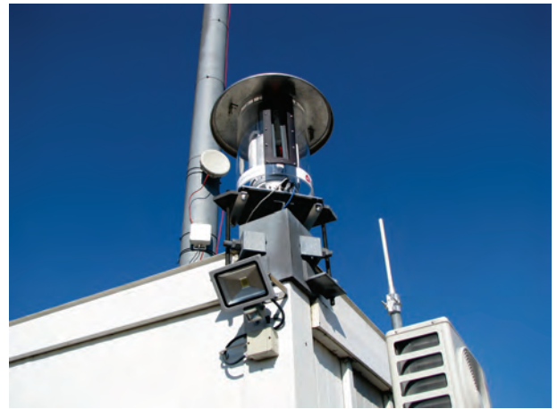
Figure A5. Another mounting example from a DMT's monitoring project.
